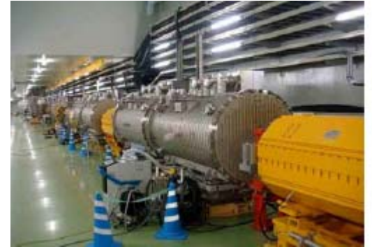
Installed Kicker Magnet
