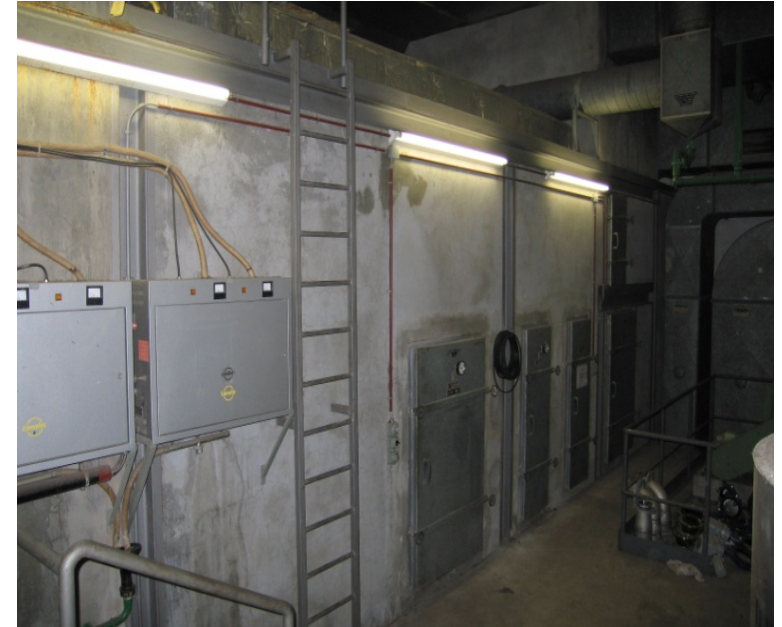
One of the 4 AHU's to replaced
