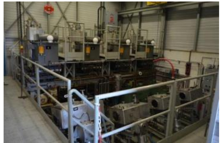
PS injection kicker generators
