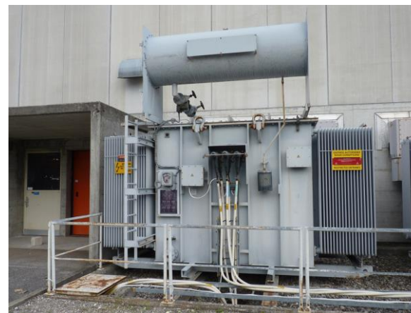
Oil Transformer Type
