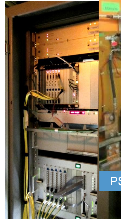
Acquisition & Processing Rack
