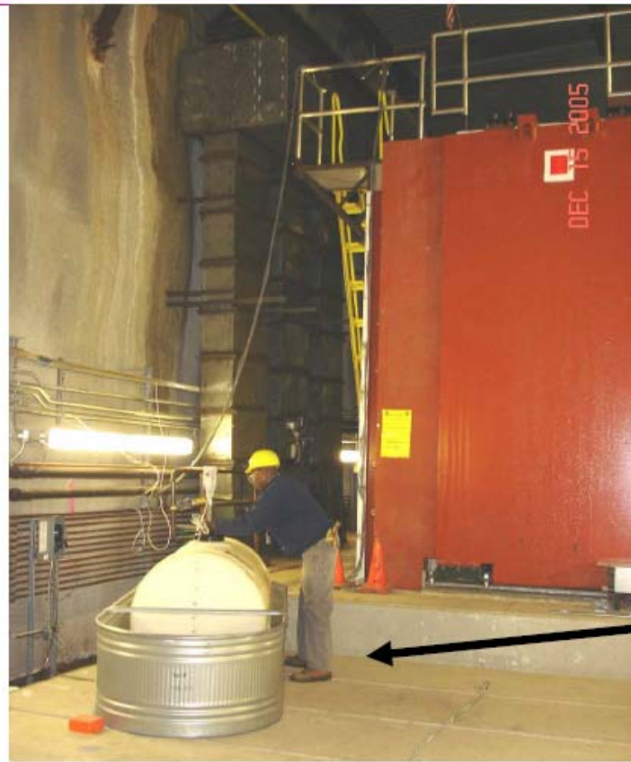
Chiller Condensate Tank
