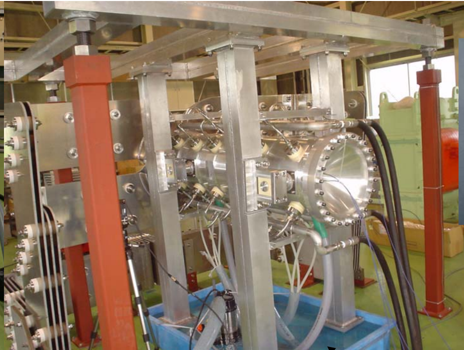
Water circulation system
