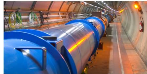
Continuous magnet line installed in the 27 km LHC tunnel, 2006
