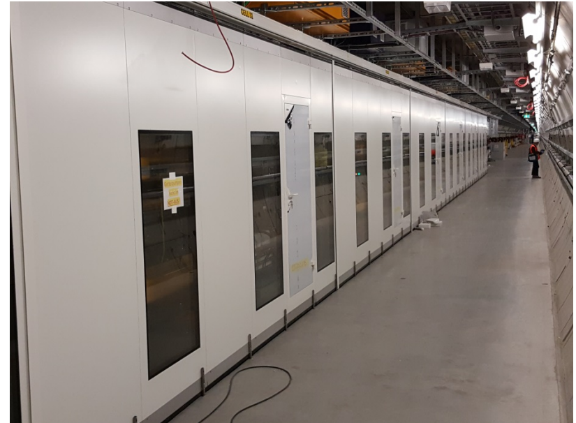
With Air Condition Enclosure 20.5.2016
