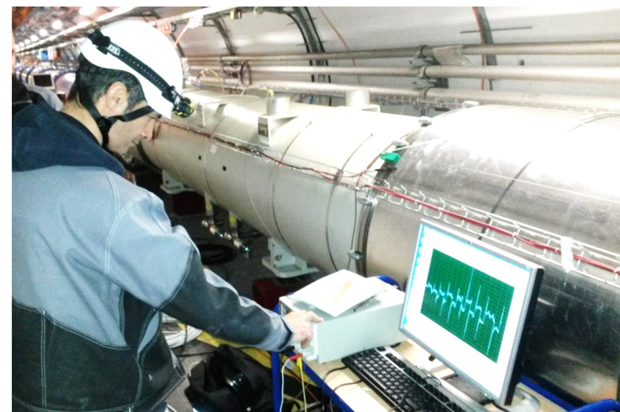
Fault localization procedure: the fault needs to be localized with a precision of 20 cm in a powering segment of 3 km.
