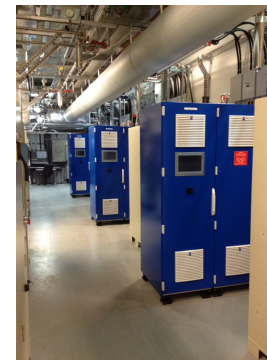
Fig.8 Dipole cabinets on site
