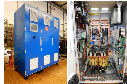
Fig.6 & Fig.7 Dipole converter (outside and inside view)
