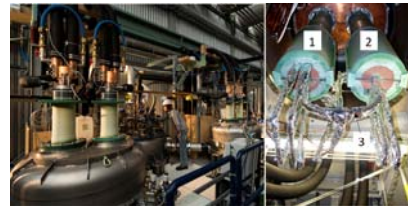
Left: picture of the test facility CuLTka showing two test cryostats (left and right) and the valve box (center). Right: test setup located within a test cryostat with two current leads (1,2) connected by a short circuit bus bar (3).
