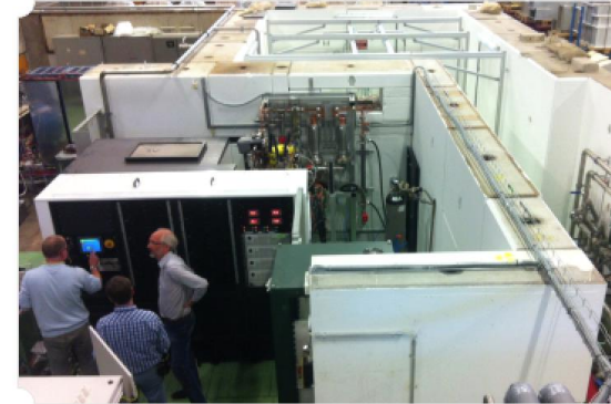
Example of X-band test facility at CERN
