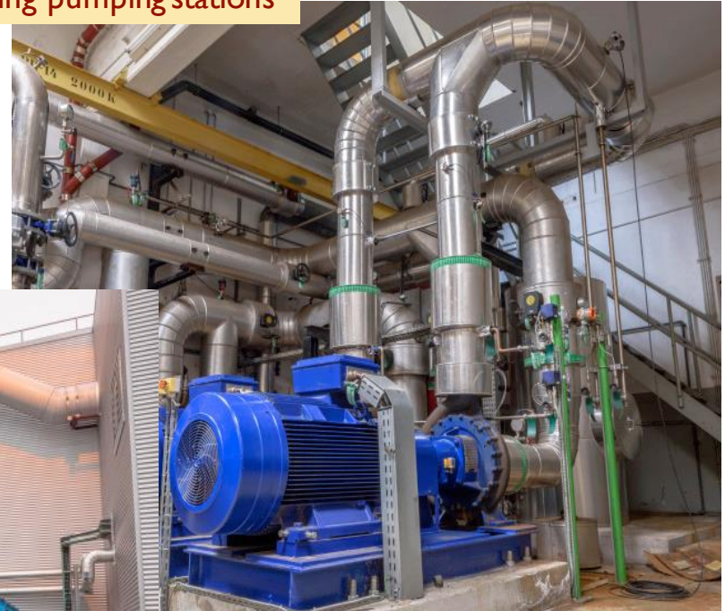
Cooling pumping stations
