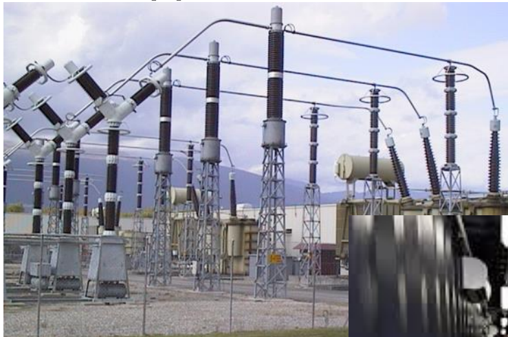
400/18kV 90MVA transformers for the SPS pulsed loads
