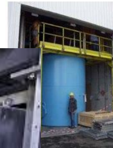
Compressor station and liquid nitrogen pre-cooler
