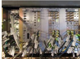
Electronics Low-level RF systems
