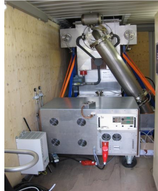
Reactor & power supply
