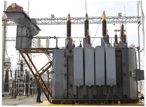
Fig. 2 The testing transformer
