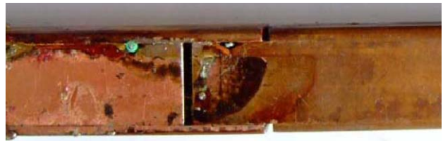
Figure 2: An intentionally poorly made bus joint, illustrating the possibility of a gap in the copper stabilizer.
