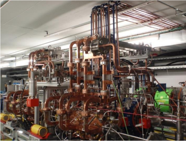
Connection by waveguide to the gallery
