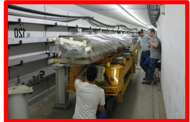
DESY conventional-magnet installation Capacity: ??? Eq. height: ???
