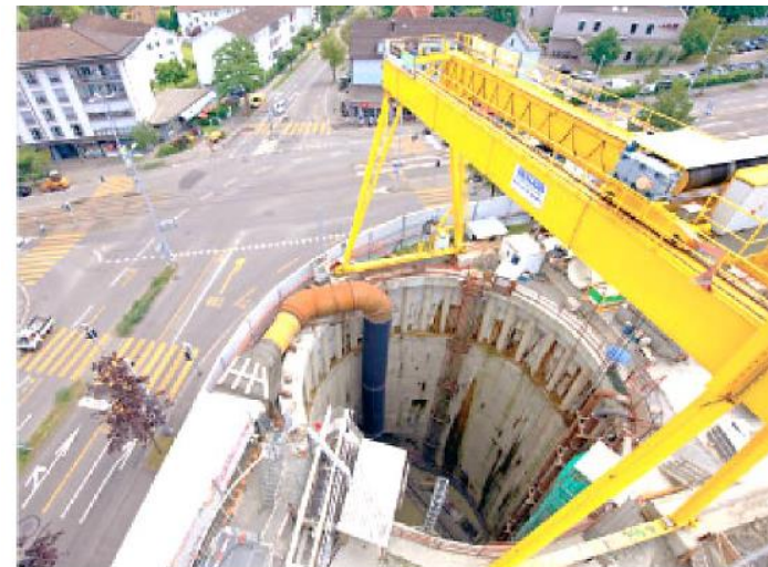
Figure 27: Shaft Brunnenhof of SBB Zürich cross line, 23 m in diameter, 42 m depth, in Moraine and Molasse (out of this shaft started a shielded multi-mode TBM with 13 m diameter)
