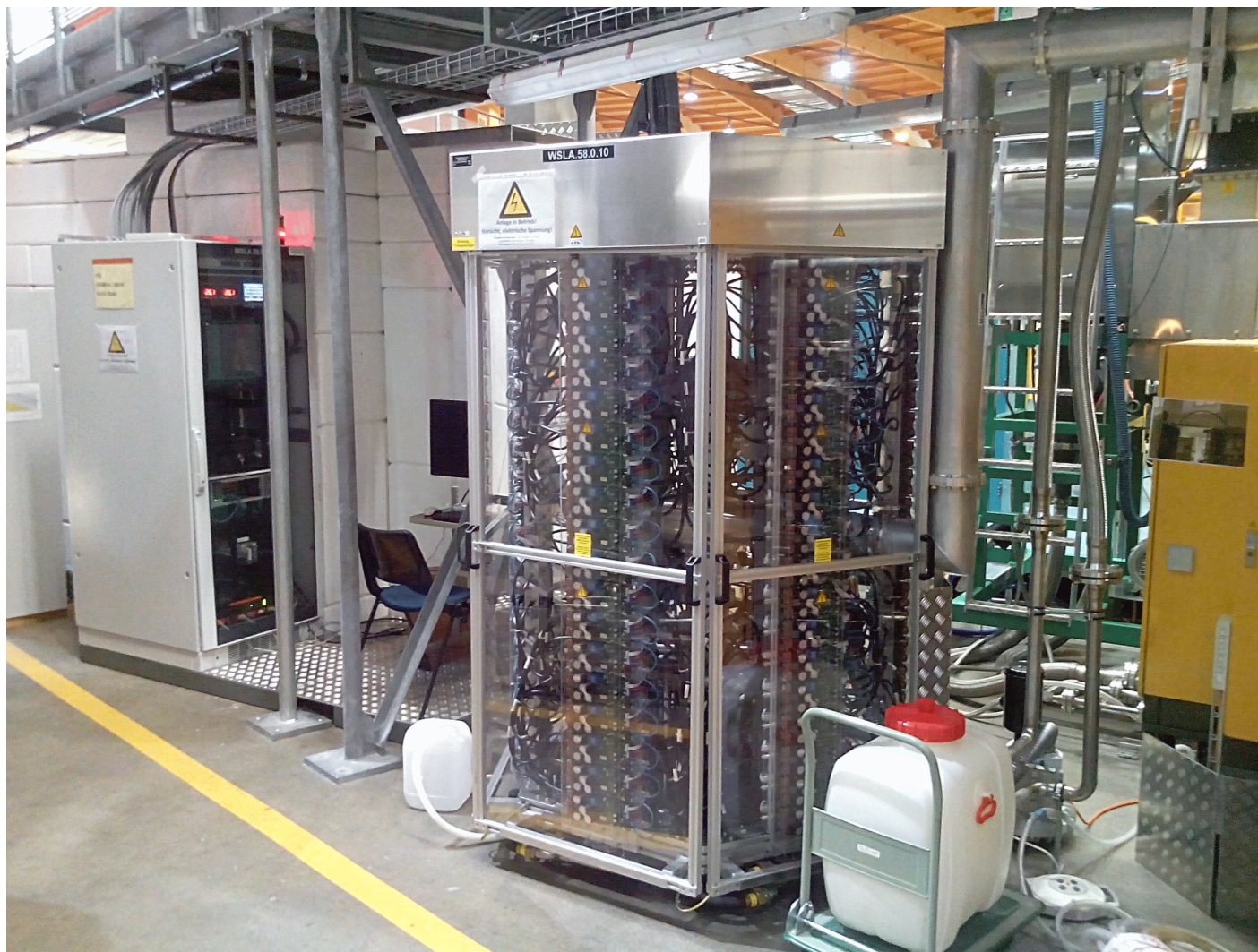
65kW 500MHz Amplifier System Installed in SLS.
