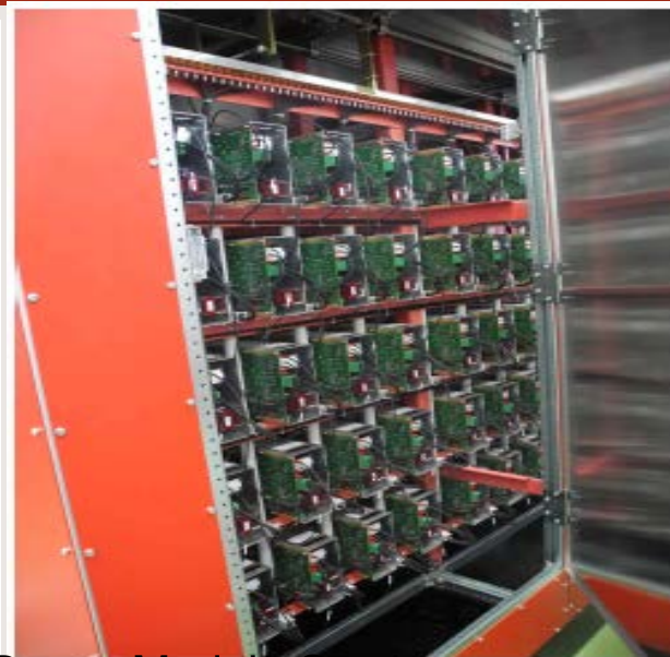
Power Module Section
