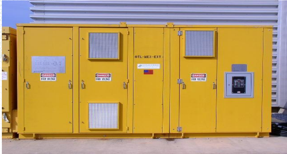
1.5MVA Transformer 13.8kV/2.1kV 3Φ
