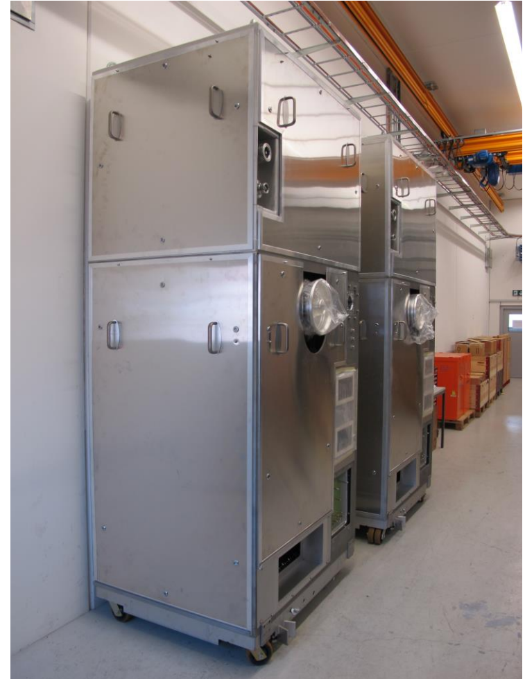
2 x 1MW Amplifiers assembled
