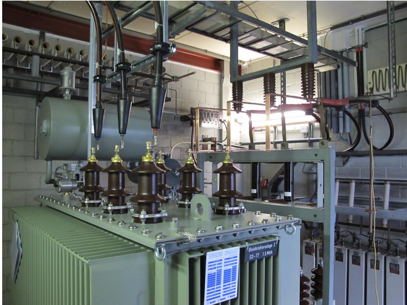
Transformer installed during shutdown 2016
