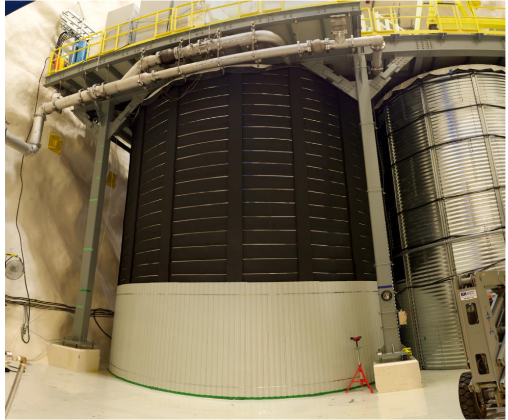
Shield Tank and emergency vent lines, tank was filled with water Oct 2015
