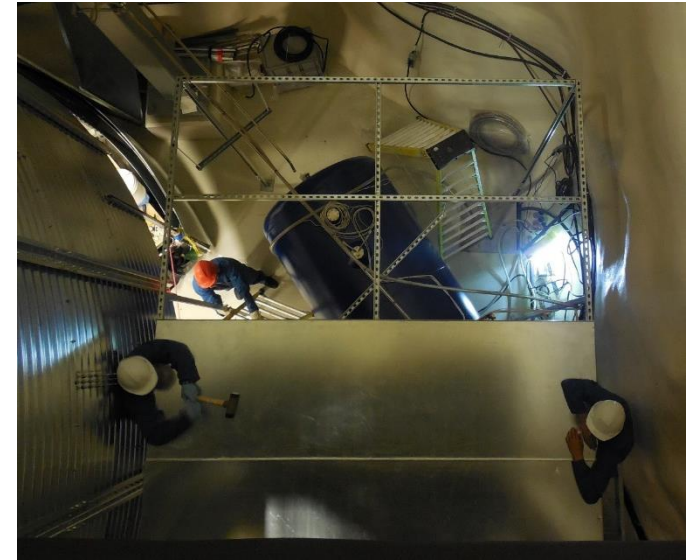
LN 2 -cooled storage dewar underground
