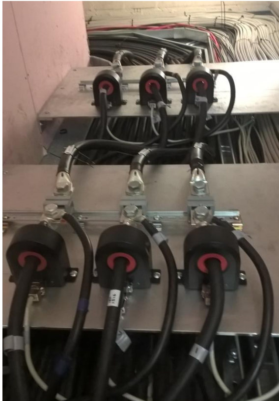
Centre & Match DCCTs mounted under stairs
