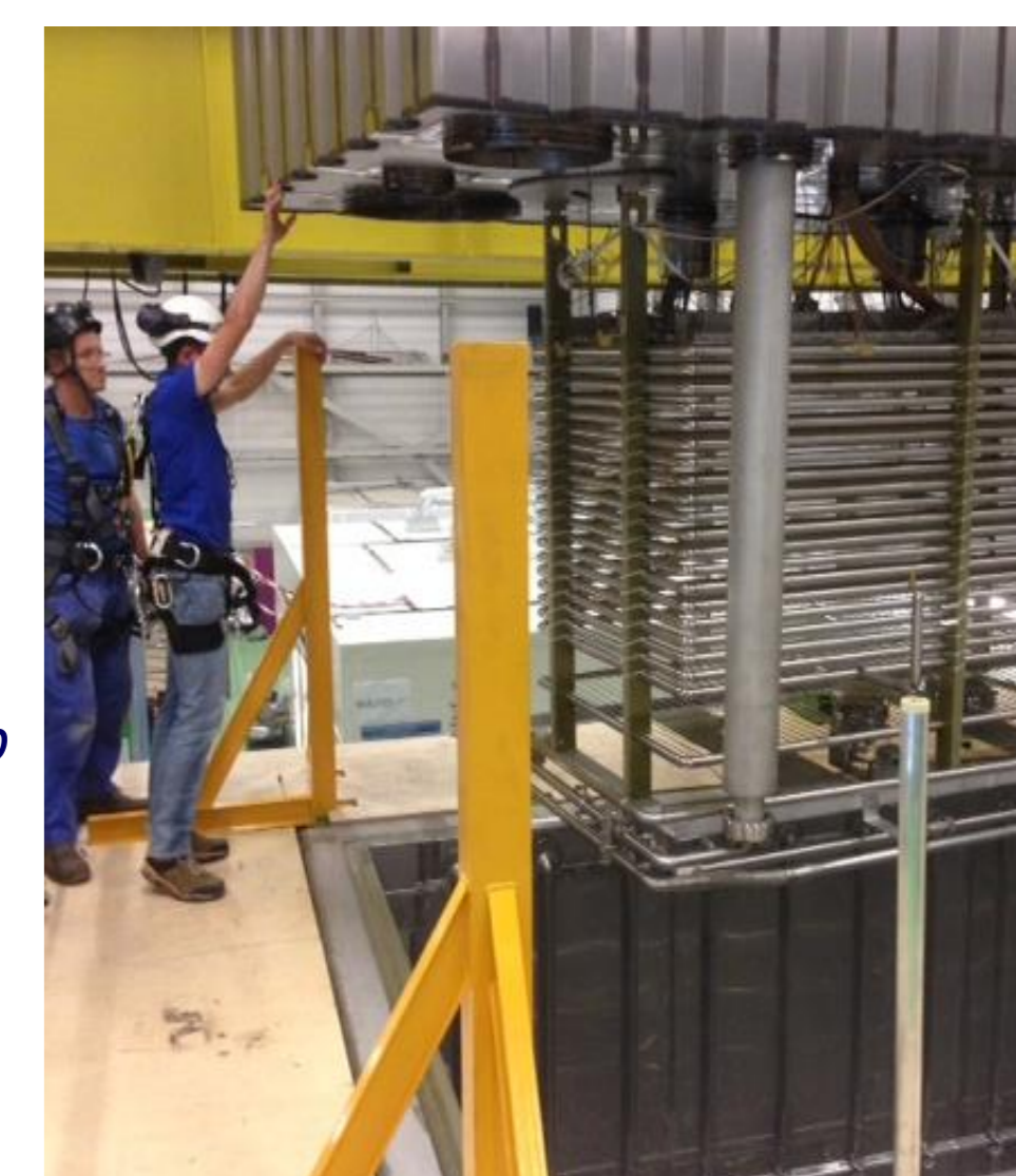
WA105 prototype - Top Cap insertion in the Cryostat
