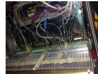
installation of front end electronics
