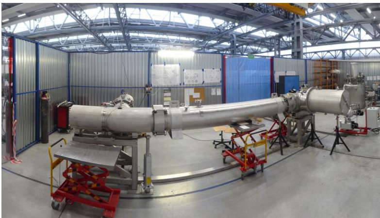
First cryogenic bypass line ready for shipment
