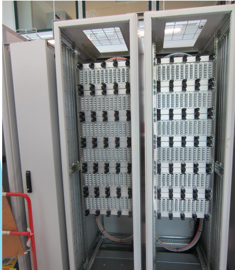
47U racks Patch cords not yet installed
