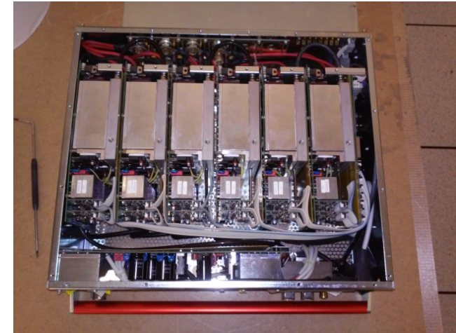
View of opened LV power supply cooling block to be replaced seen at bottom right
