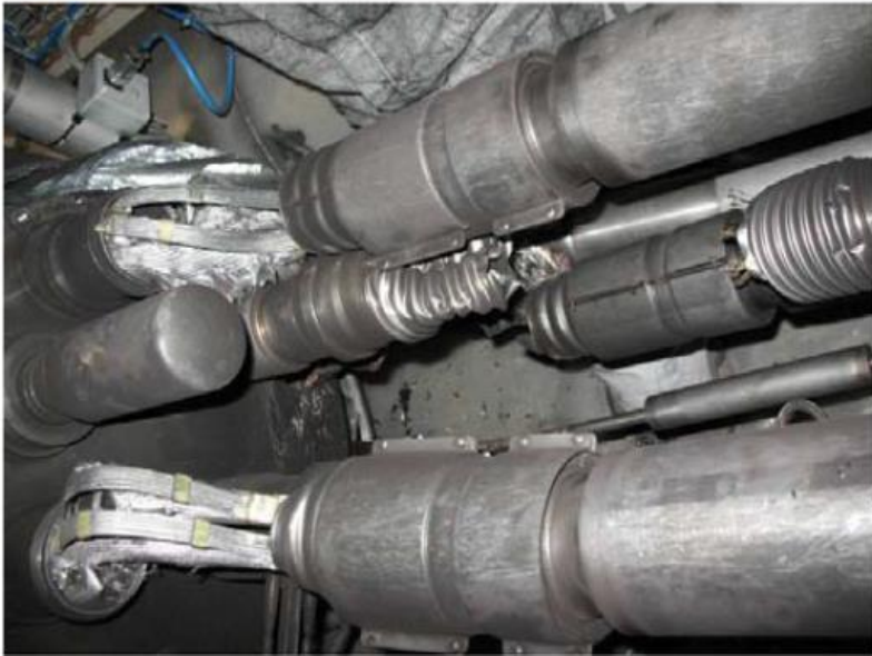
Damage to interconnection QBQI.27R3 by excess extension
