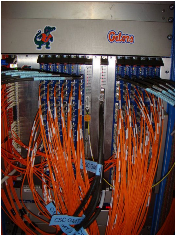
Figure 3: Front View of the CSC Track Finder crate
