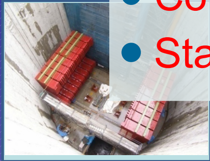
UA1 magnet donated From CERN installed
