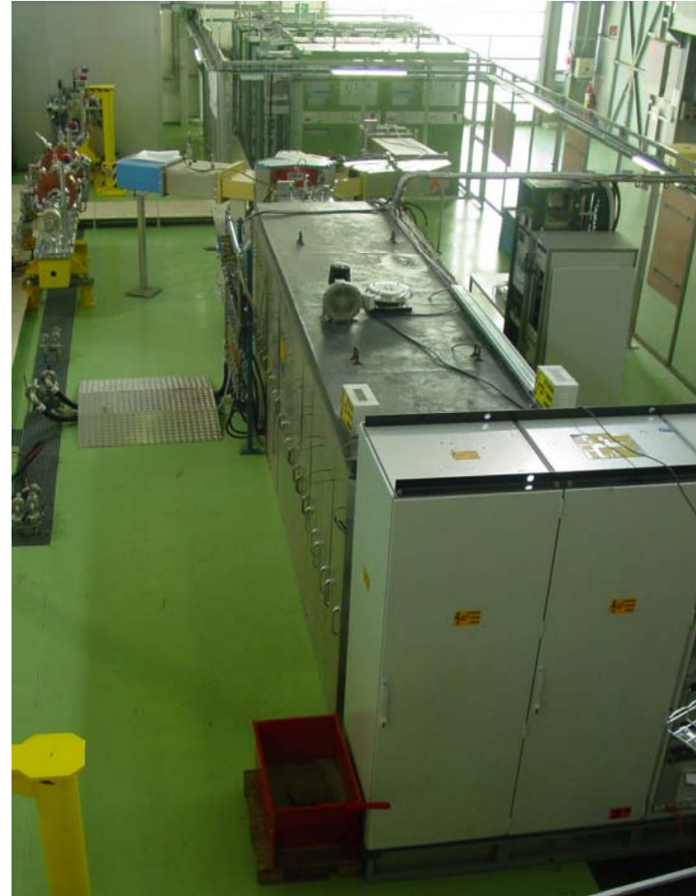
LEP-type klystron and prototype modulator under test
