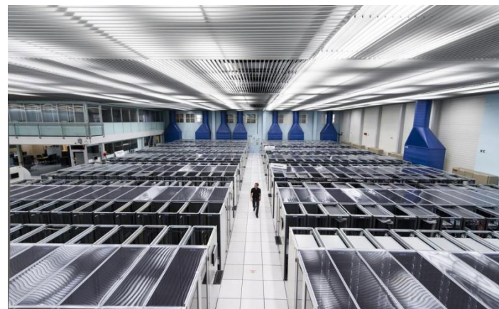
CERN Data Centre, 2016
