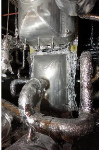
Heat exchanger tapings (taken out)
