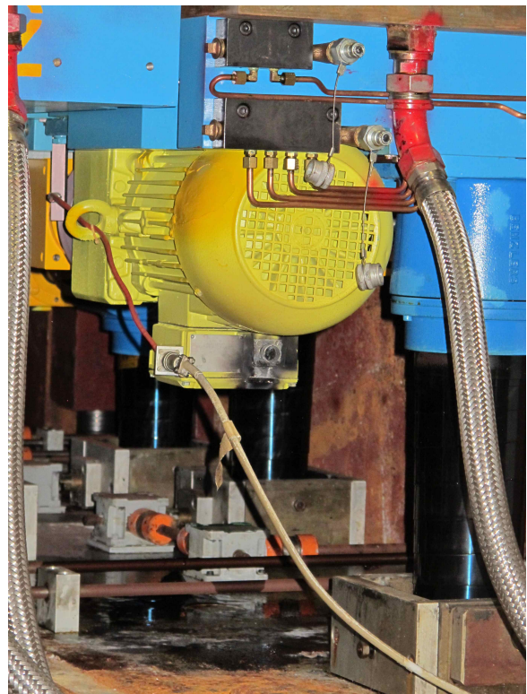
Figure 2: Photo of one of the damaged motors. The signs of the short circuit at the connector are clearly visible.
