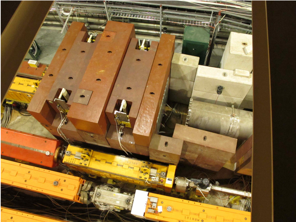
Figure 3: Photo from the TCC2 overhead crane showing the M2 TAX assembly. The TAX blocks are inside the iron shielding
