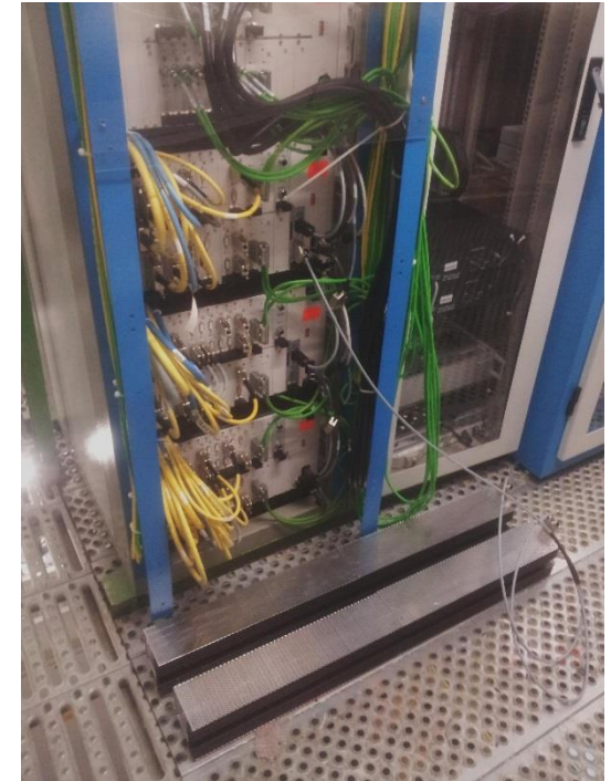
Remote online tests and PLC tests.
