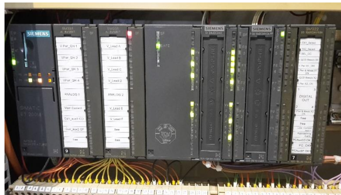
Example of a PLC
