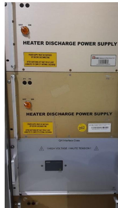
Heater discharge power supplies
