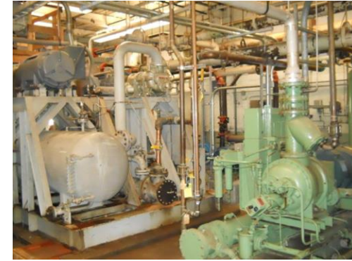
Mycomm and Sullair 350 compressors
