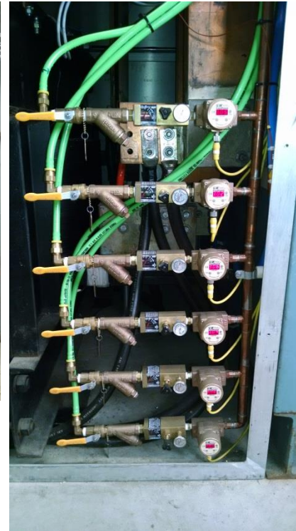
Plumbing and flow gauges with signal acquisition for IGBT water cooling and monitoring.
