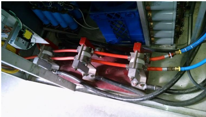
Existing three water-cooled free-wheeling diodes in parallel.
