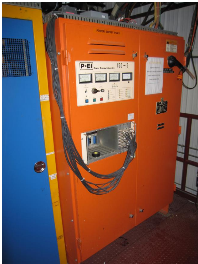
150 kW Power Energy Industries (PEI) PS module (left)
