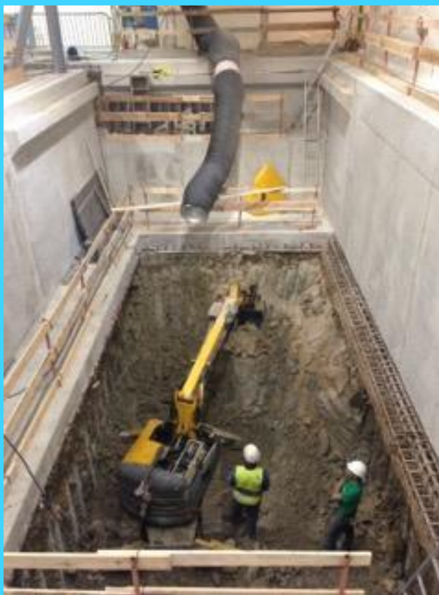
Ref. Construction: H. Botella, R. Morton, E. Perez Duenas, Safety: E. Paulat
