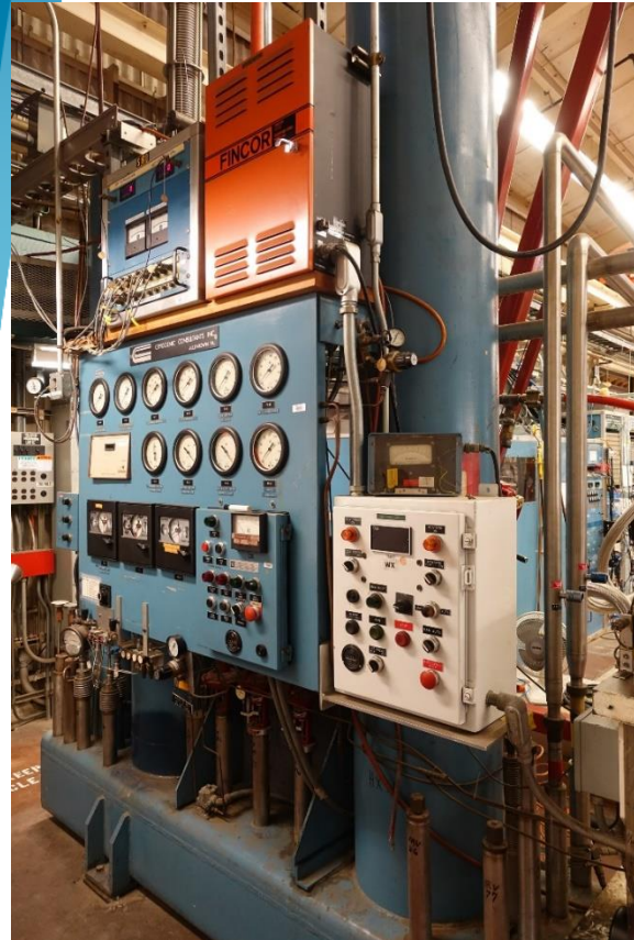
Liquifier control panel
