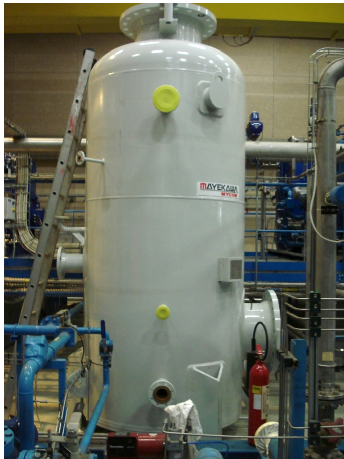
NEW Primary Oil Removal System
