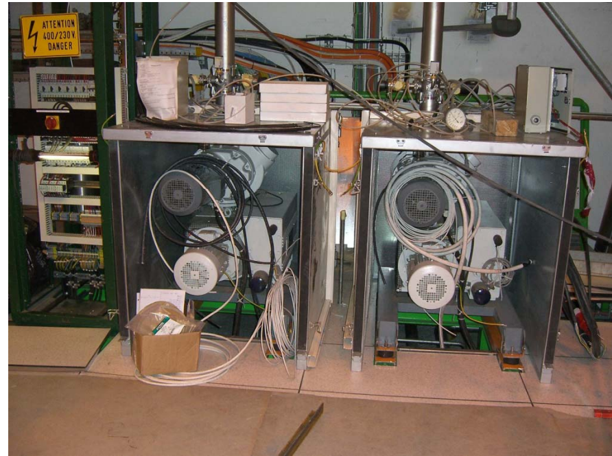
Primary vacuum pump and rack
