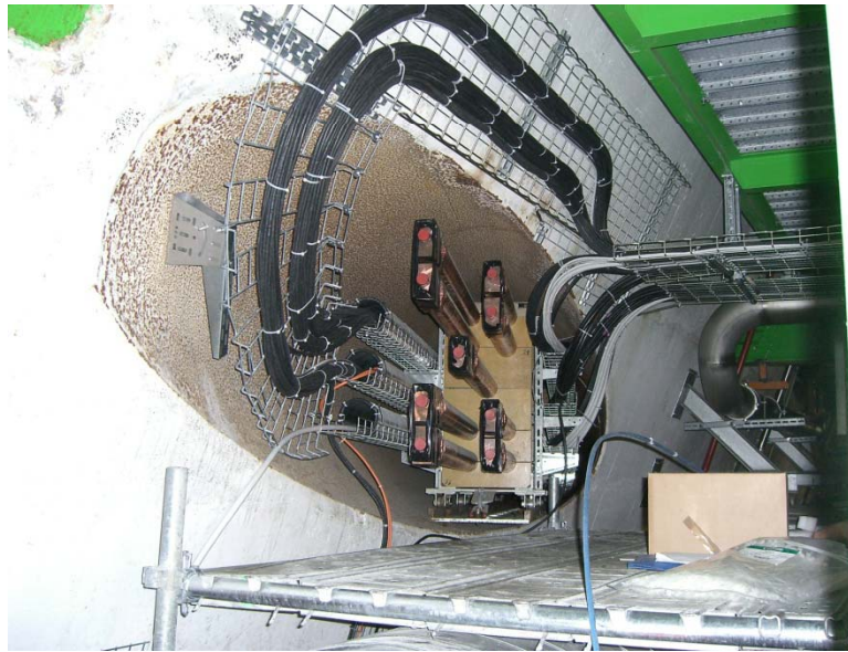
Instrumentation Cables UX Side
