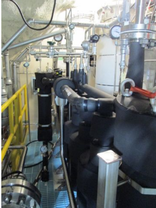
Scintillator purification plant underground
