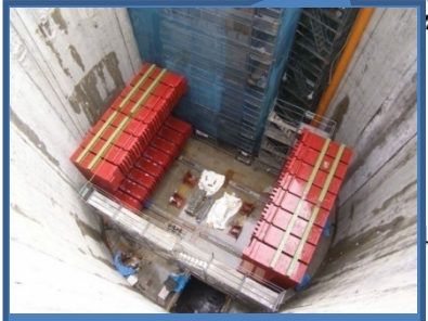
T2K Near Detector In preparation
