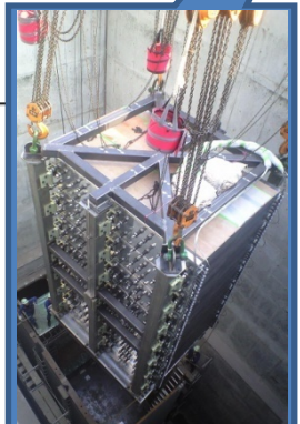
Beam dump installed
