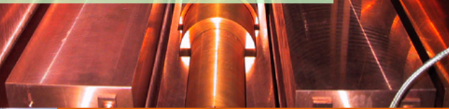
detectors during installation; in the central and right up detectors the new shaped Cu shield surrounding light guides (acting also as optical windows) and PMTs was not yet applied
