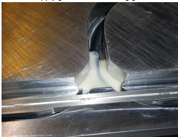
Figure 21 Strain relief of the cables of the light bars
